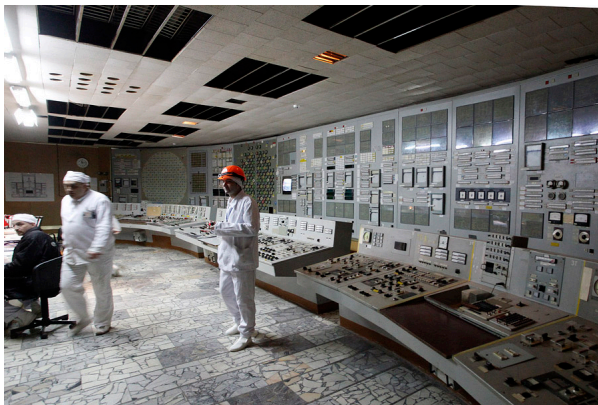
The control room, Reactor 4, Chernobyl Nuclear Power Station
